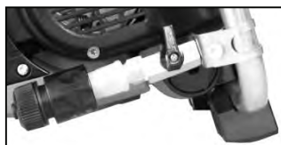
water supply closed (valve lever across)
